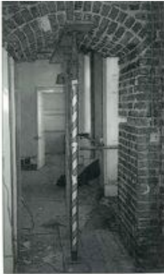
Above: Emergency propping installed to support the brick arch following decay of timber
